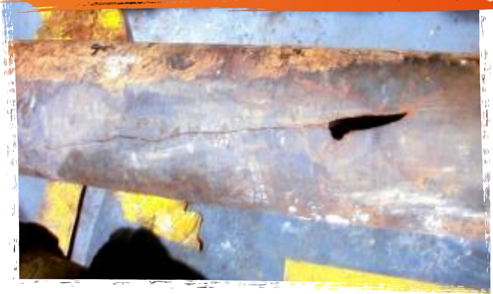
Ageing gas pipes today
