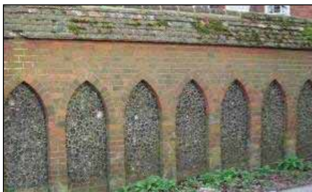
Blind Gothic arches set into red brick, infilled with flint, and surmounted by a tiled roof create a charming boundary wall to a Victorian house on Winter Hill.
