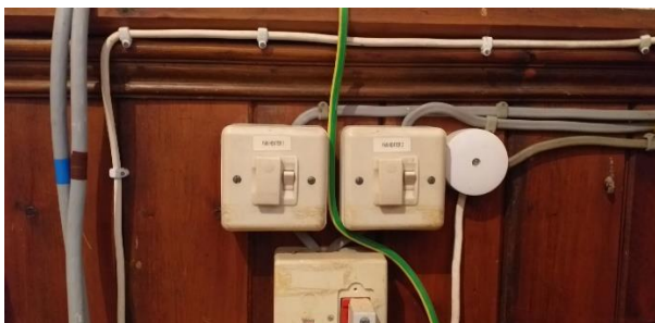
Heater switches in the vestry.
